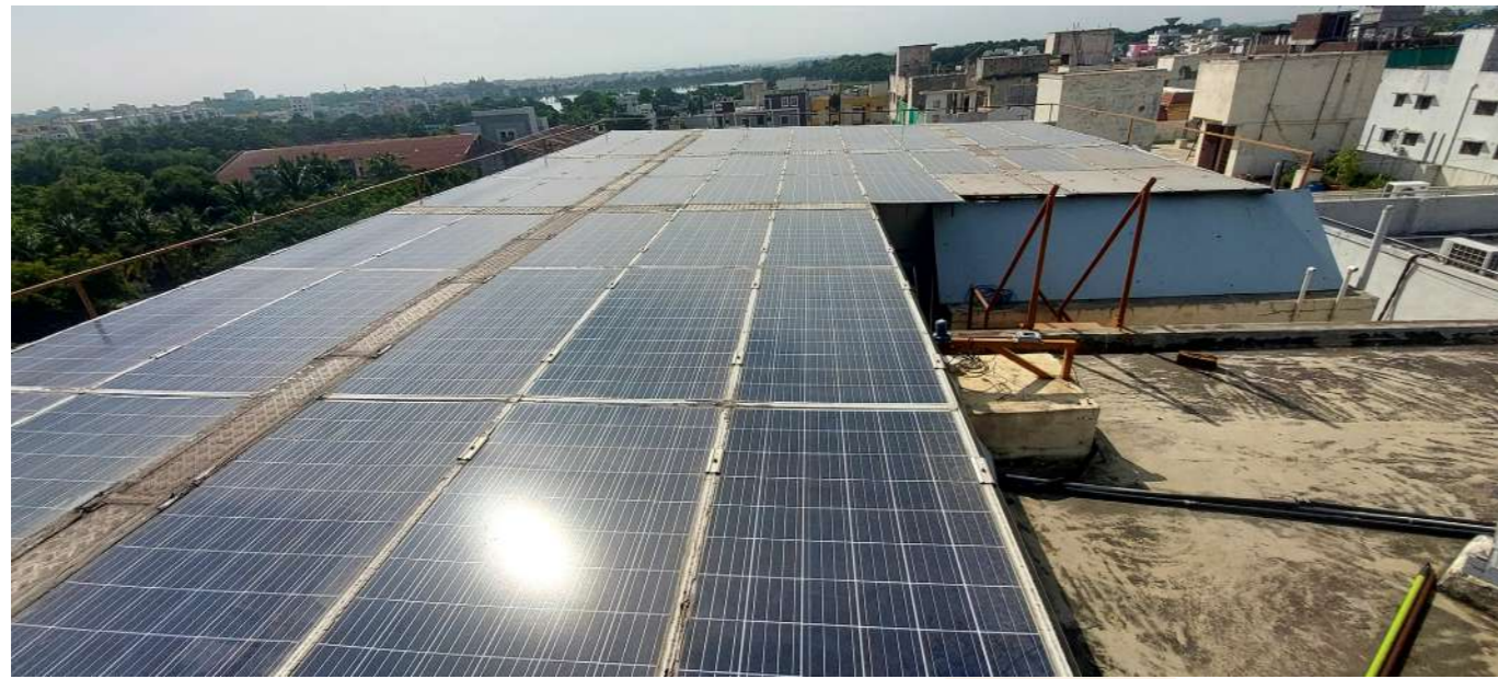
Rooftop Solar, FPEL Office, Hyderabad, India
