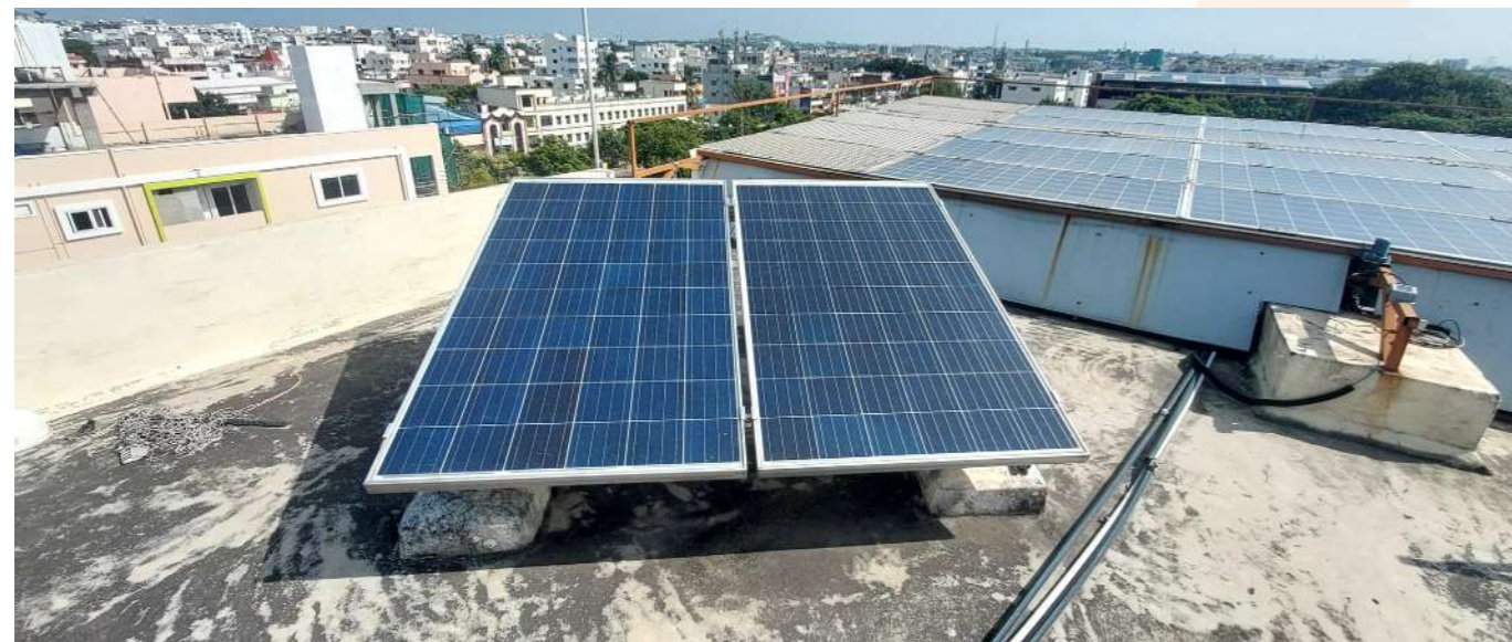
Rooftop Solar, FPEL Office, Hyderabad, India
